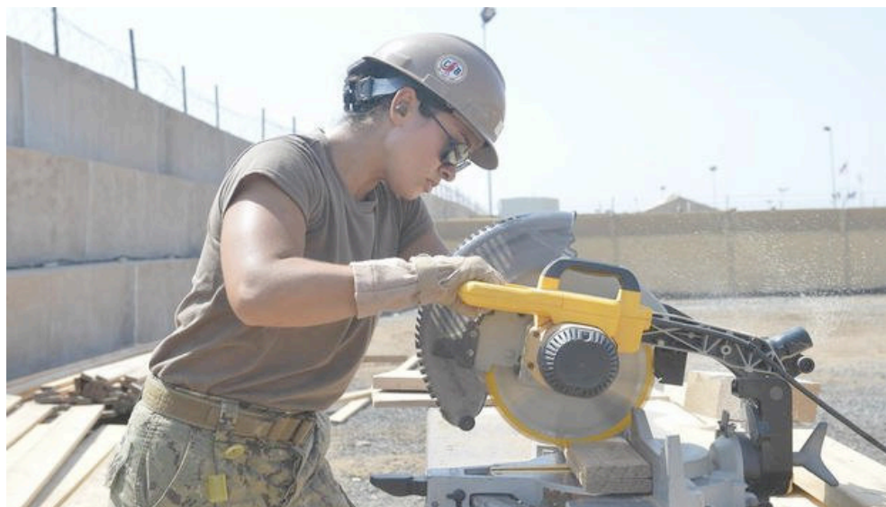
Construction Electrician Constructionman Stephanie N. Bugaski from Naval Mobile Construction Battalion 133, deployed with the Combined Joint Task Force - Horn of Africa, cuts wood new bus stops onboard Camp Lemonnier. (U.S. Navy photo by Mass Communication Specialist Jared E. Walker)
